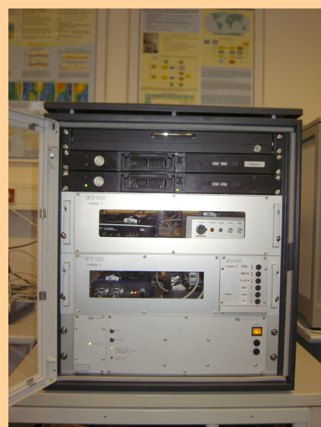
Figure 2a: GFZ GSS (Geodetic Sensor Station), test installation at Potsdam
