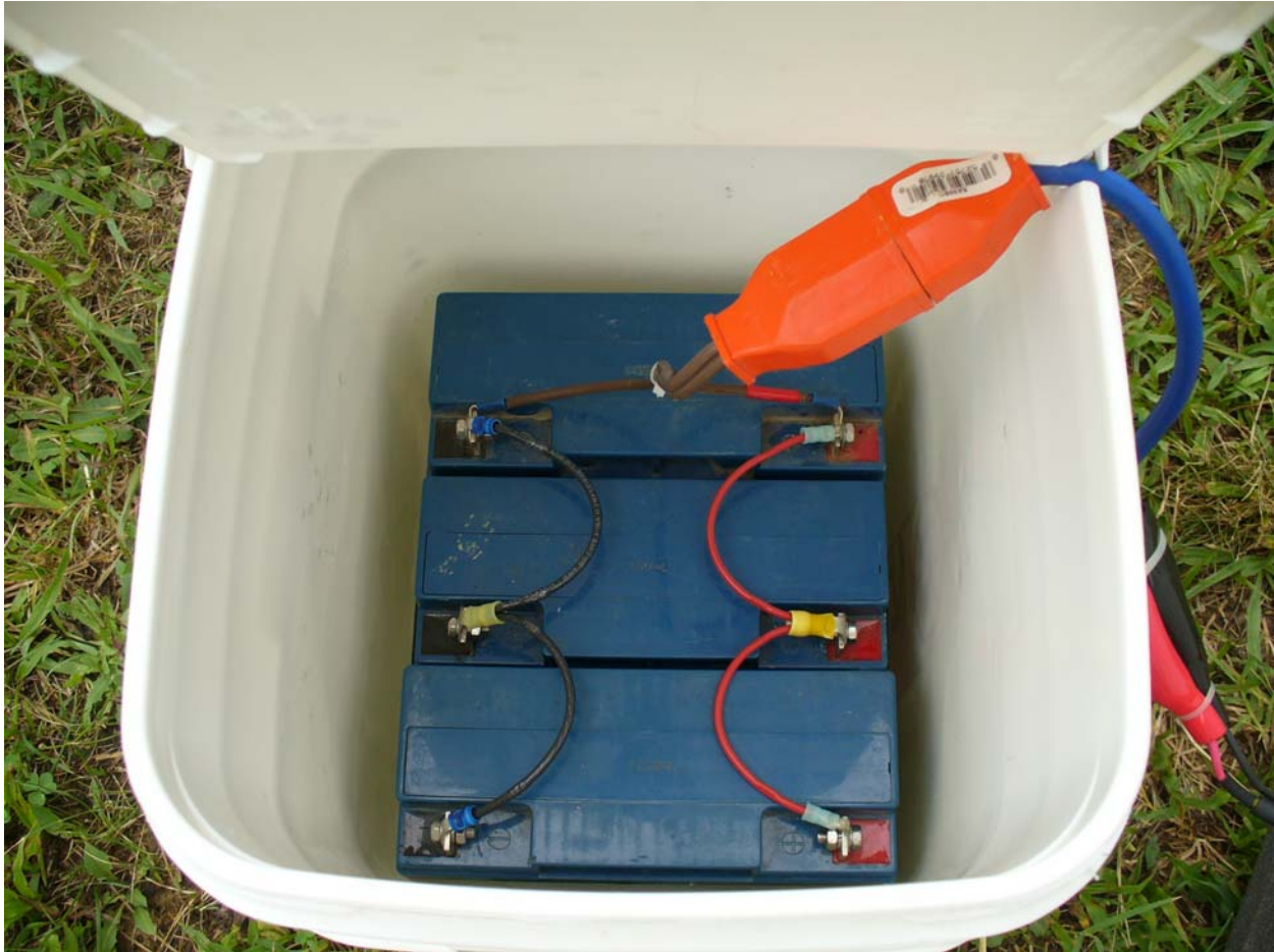
Figure 8.3. Three 18-Ah “gel cell” batteries taped together and wired in a parallel circuit fit nicely in the bottom of the bucket. Three-prong connectors were used to prevent damage to GNSS receiver by accidentally reversing the polarity when connecting the batteries.
