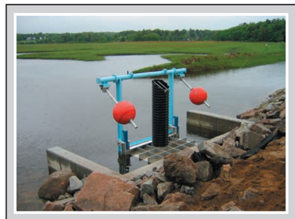
New box culvert and self-regulating tide gate at Drakes Island Marsh, near the Wells NERR.
