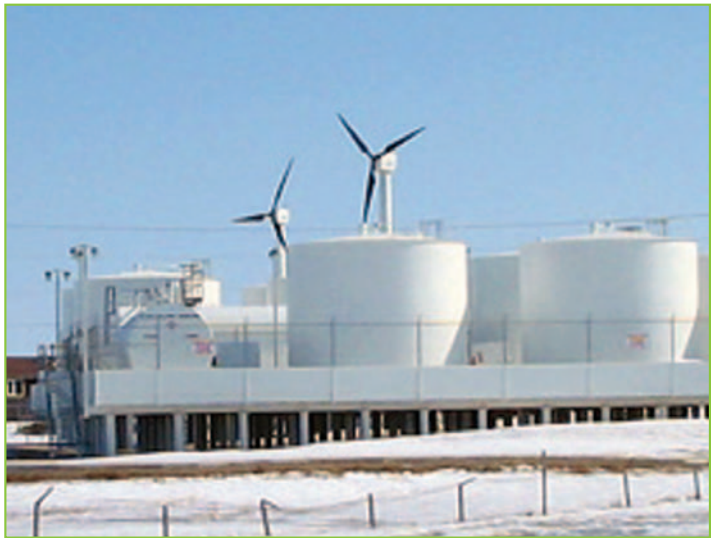
Two of three wind turbines can be seen over the bulk fuel tanks of the Kasigluk Power System. Ian Baring-Gould/PIX16097.
