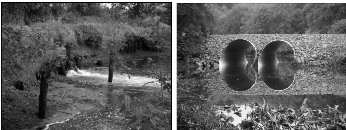
Figure 3. Tide gate at Kandoll Farm before (left) and after (right) culvert replacement.
