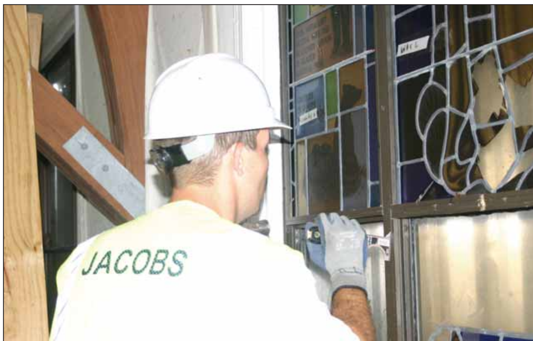
A Willet Hauser employee carefully removes a stained glass window at the Chapel. All of the stained glass windows have been removed and shipped to Philadelphia for repair and restoration.
