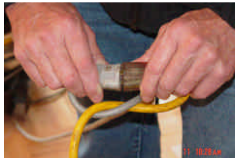
Path to ground not continuous. Snipped grounding conductor.
