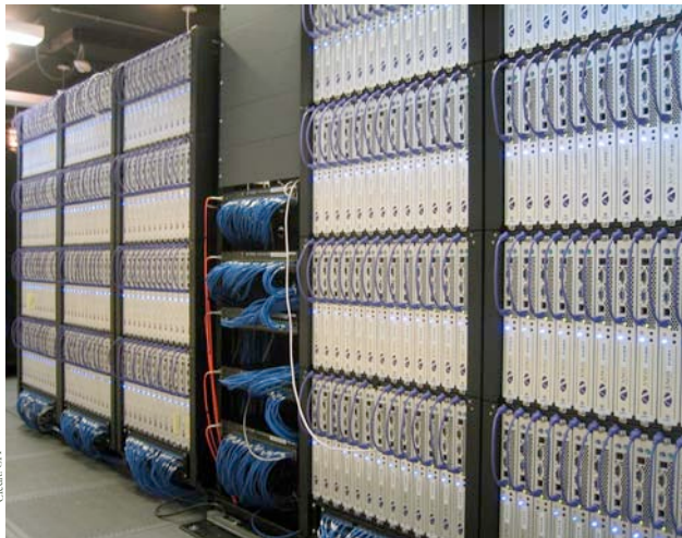
The Biowulf cluster is housed in Building 12, occupying 3,000 square feet of space. Visitors might feel they are descending into Grendel's lair, as the heat and hum of the computers grow more intense as one approaches the system through double doors secured by a retinal scanning device. A sophisticated cooling system was installed three years ago to handle the growth.
