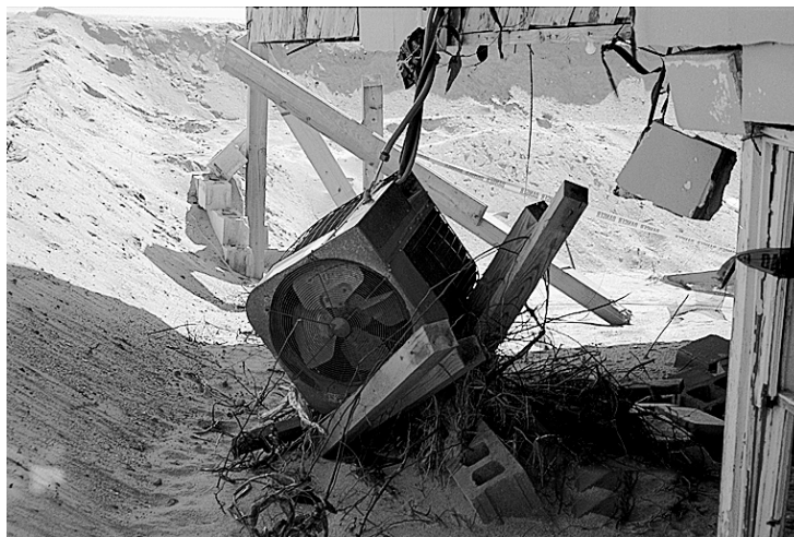
Figure 1.2.1A: Electric heat pump dislocated from its shattered wooden stand by velocity flow in a coastal area
