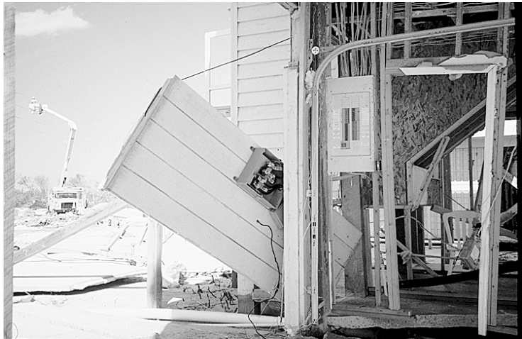
Figure 1.2.1C: Electrical panel board damaged by velocity flow in a coastal area
