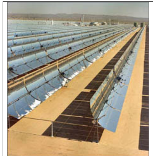
Figure 57 Parabolic-trough concentrating solar power system. Image courtesy NREL 311
