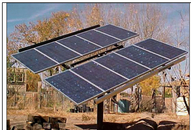
Figure 7 Solar tracking unit. Image courtesy Northern Arizona Wind and Sun 40
