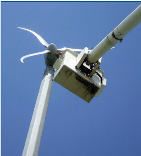
A Skystream turbine was installed at Kansas State as part of the Kansas Wind for Schools program. Ruth Douglas Miller/PIX16025
