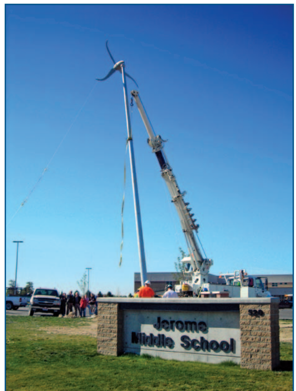
A Skystream turbine is installed at Jerome Middle School in Idaho as part of WPA's Wind for Schools program. Stephanie Lively, Boise State University/PIX16146.
