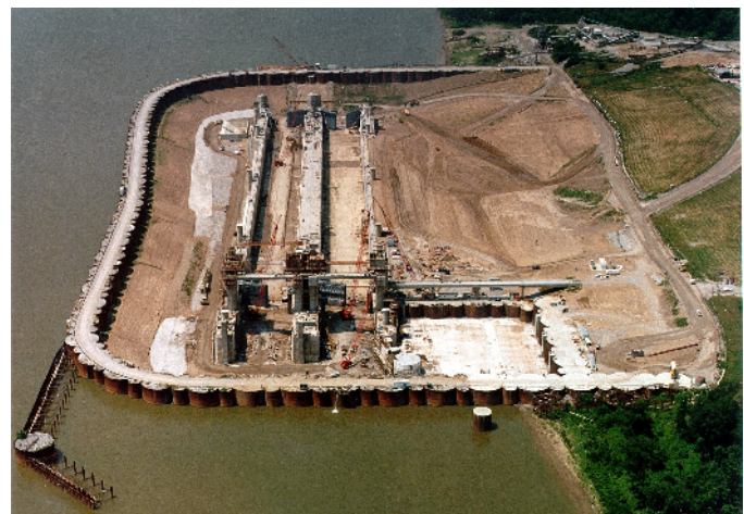
Navigation locks and dam under construction. The budget proposes to spend $73 million in 2004 to rebuild Olmsted locks and dam to reduce delays on the Ohio River. Construction work began in 1991 and originally was scheduled to be finished by 2006. At this point, it may not be completed until 2010.
