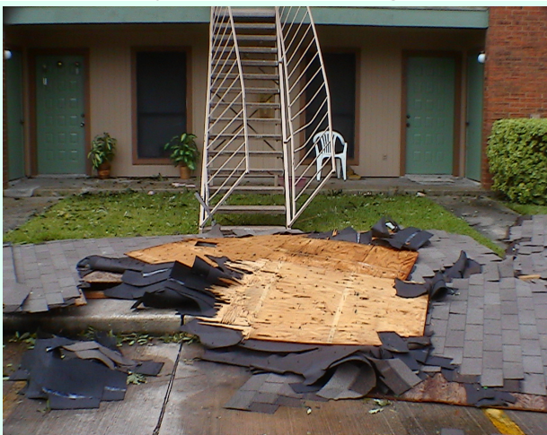
Damage to apartment buildings in Port Arthur, TX (photo by Joe Catalina)
