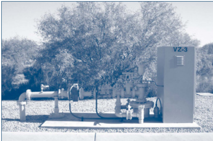
A reclaimed water recharge well in Phoenix, AZ. SOURCE: Andy Terrey, City of Phoenix.
