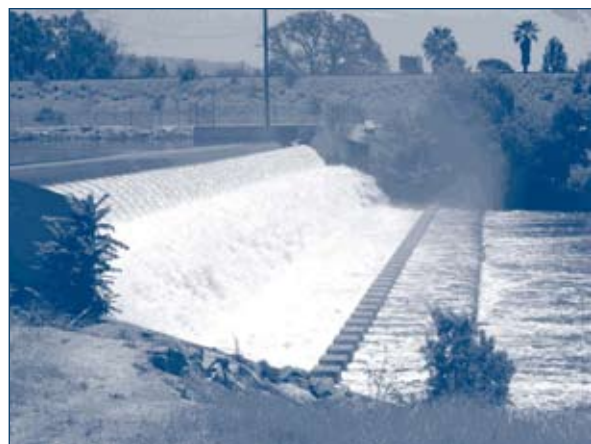
Rubber dam owned by Water Replenishment District of Southern California. Inflated (top) and deflated (bottom).
