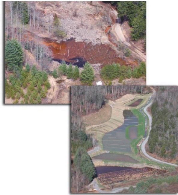
Pollution and sediment used to drain into Ely Creek in Lee County (top). Now water quality in the stream has improved due in part to a wetland that was constructed to the left of the stream (bottom).
