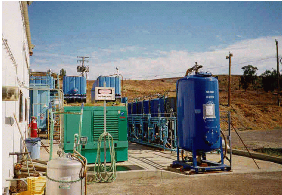
Treatment System, Casmalia Resources
