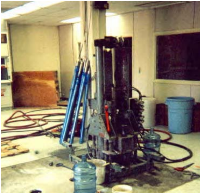
Figure 4-5. Indoor Vibra-Push Rig (LD Geoprobe® Series) Used in the Engineering Support Building
