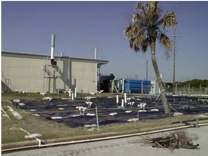
Figure 3-2. Resistive Heating System in Operation at Launch Complex 34
