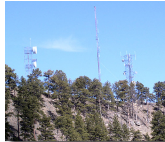
Communication facilities located on private property atop North (Windy) Ridge are among the developments potentially threatened by wildland fire.
