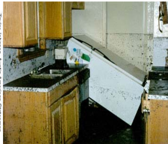
Figure 1.2 October 1998 – Flood waters in caused extensive damage in this Williamson Creek home.
