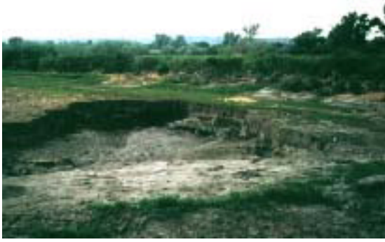
When the Yellowstone River threatened to reroute its course through the Canyon Creek irrigation canal, flooding part of Billings, NRCS employees designed a system to protect the canal and ensure the Yellowstone remains in its banks.
