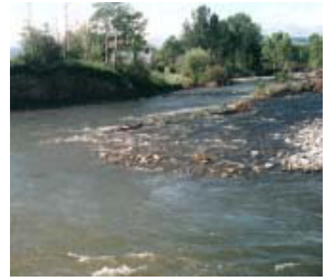
EWP funds were used on the Lower Middle Canal on the Gallatin River to protect and rebuild the irrigation inlet area damaged by flood waters.
