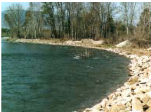
Rock riprap was used on the Bitterroot River to protect a business near Florence from erosion.
