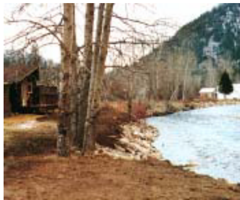
Rock riprap on Lolo Creek protects property, a bridge, and a highway from flood damages.
