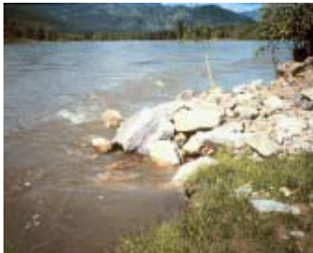
A series of bending wiers and bank protection were used to stabilize the banks of the Clark Fork River and allow it to move back toward its original channel.
