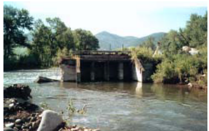
The Highline irrigation canal on the Gallatin River suffered severe erosion from flooding. EWP funds were used to repair the inlet area and canal and Emergency Conservation Program funds from the Farm Service Agency were used to repair the inlet structure.
