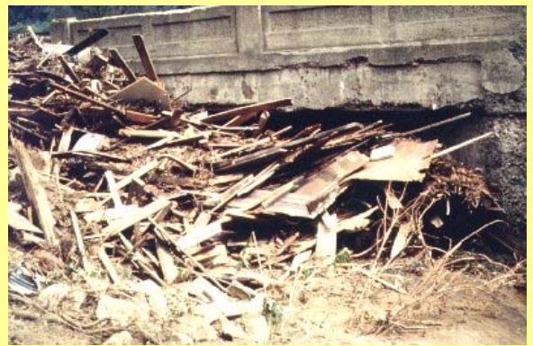
Fig. 2.3-1 Debris Blockage of a Bridge
