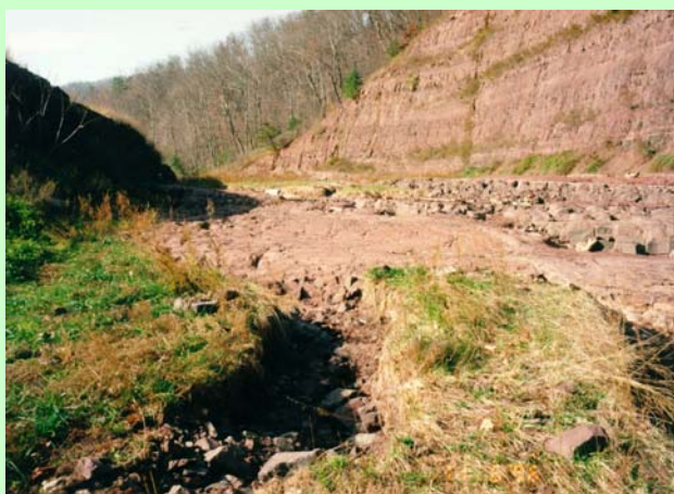
Fig. 2.3-12 Emergency Spillway Damage, Switzer Dam, Dry River, VA
