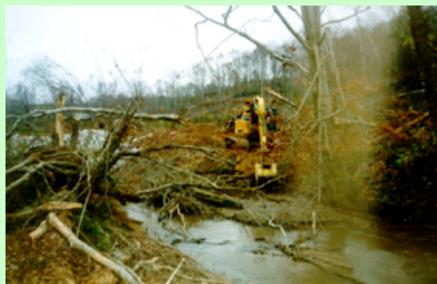
Fig. 2.3-2 Debris Removal Using Heavy Equipment (backhoe), Bethel Road Site, Hall County, GA
