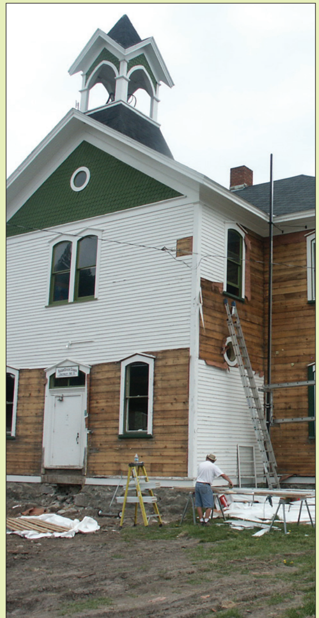
Work on the Basin School includes re-siding walls and adding energy-efficient windows to the 100-year-old structure. About 15 students attend the school.
