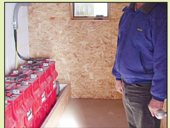
Batteries at the motel provide backup power.
