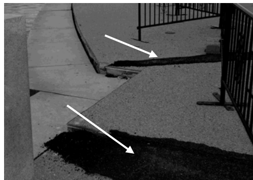
Temporary repairs have been made where settlement has become a tripping hazard to the public.
