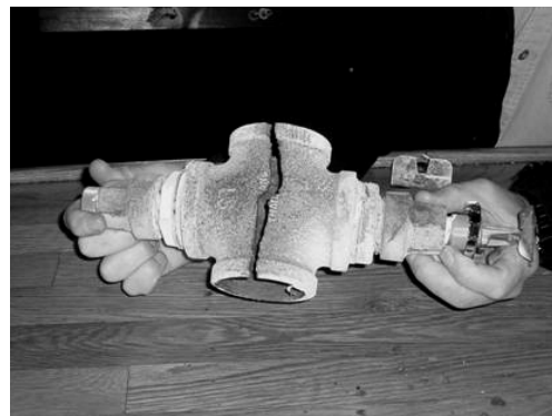
A cracked fire suppression valve, which has been replaced, reflects the current condition of similar component deterioration.
