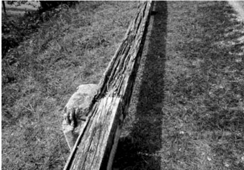
Rotting timber guardrails cannot withstand vehicle impact and provide a false sense of security.
