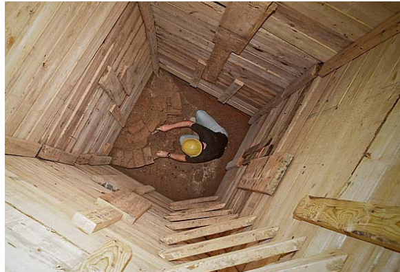
Excavation of a well at the former home of President George Washington, Independence NHP
