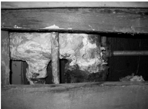
Excessive caulking has become necessary to prevent further deterioration and leakage of the sewer pipe.
