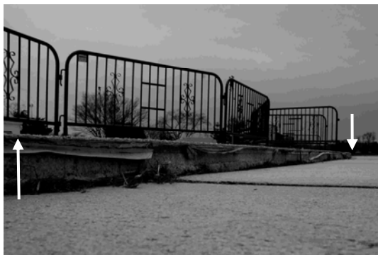
Close-up of Differential Settlement at Jefferson Plaza Seawall.
