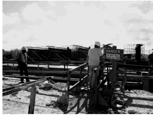
Construction of an S-357 pump station will mitigate increased water levels resulting from restoration of Shark Slough.
