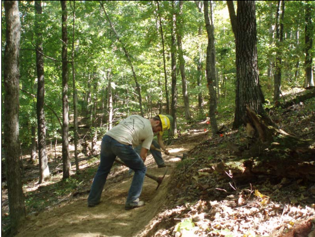
Figure 5. Trail crew digging the new trail tread for the Owl Bluff re-route.
