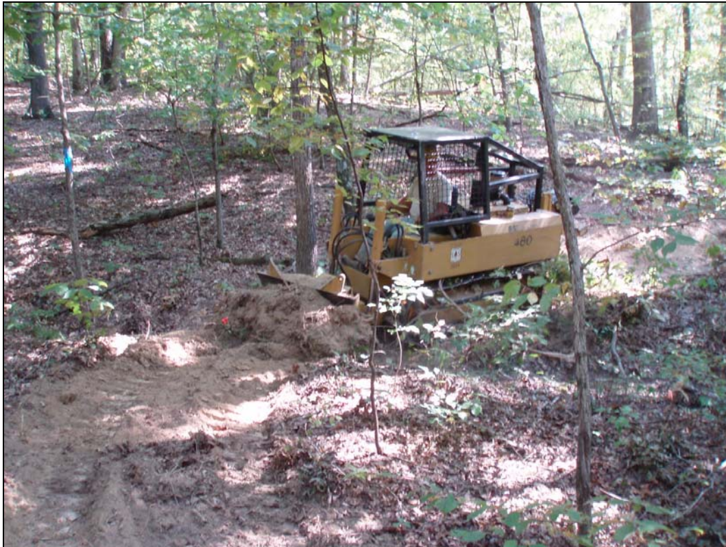
Figure 1. Sweco trail dozer being used to cut new trail tread on FS Trail 487
