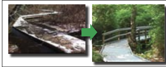
In FY 2002, $245,702 was spent to replace and construct new boardwalks throughout Cape Cod National Seashore in Massachusetts.
