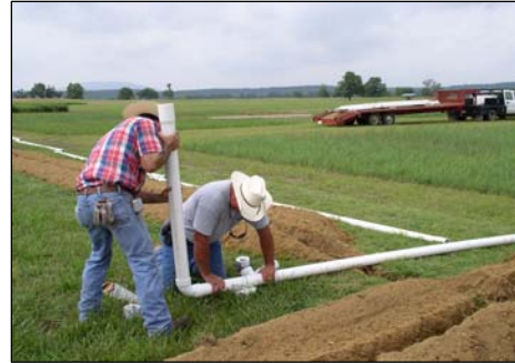
Dale Goff and Eddie Pratt installing an irrigation system on switchgrass plots
