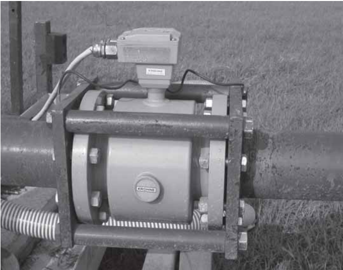
Figure 7. Magnetic-type flow meter mounted in-line on swivel pipe. Transducer with leads to tractor cab allows readout of flow rate.
