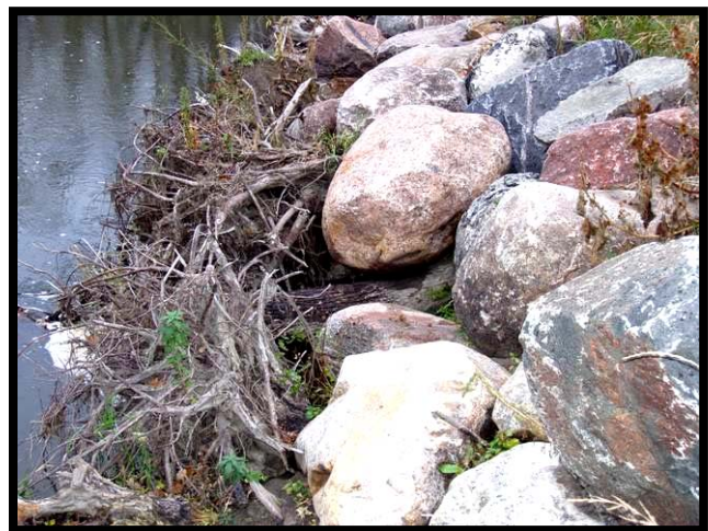
Large rocks used to protect a streambank and to hold rootwads. The river flowed between the rocks, washed the soil out from around the rootwads, and wiped out the entire bank.
