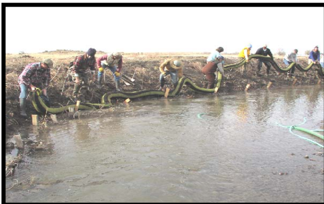
AZ workshop participants laying out a new organic soil filled sock that could either replace a willow fascine or added to it for more protection.
