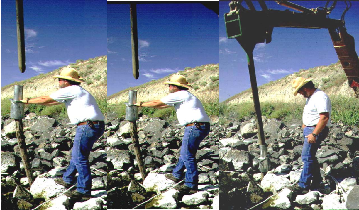
Planting a willow pole into rock riprap. In photo 1, the stinger has already punched a hole into the rock. In photo 2, the cap is placed on the pole and the stinger is guided into the hole in the top of the cap. In photo 3, the stinger pushes the pole into the pre-punched hole. The cutting will have about 1 foot sticking out of the ground when done.
