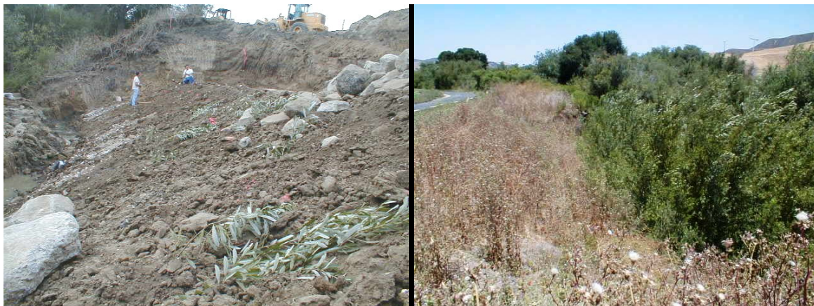
Figure 1: Vertical bundles placed behind a stone toe. Under construction and after 4 years
