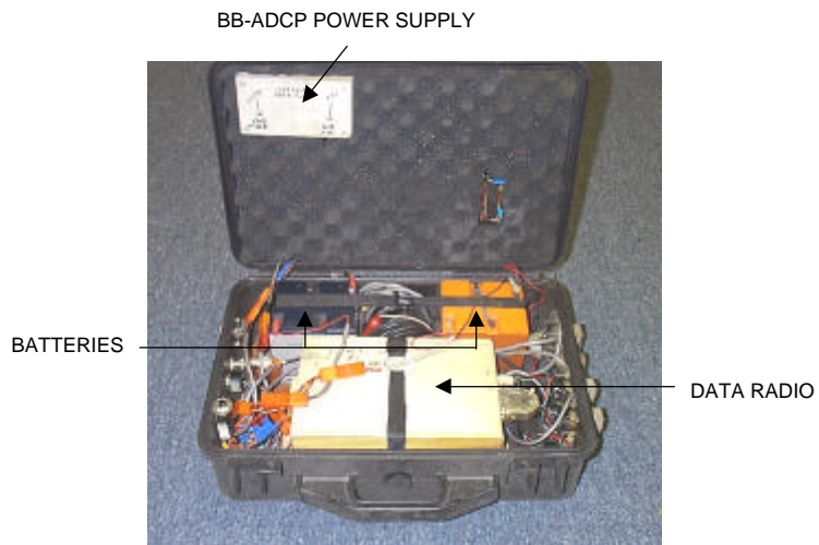
Figure 29. Waterproof case with electronics for transmitting data to the shore station.
