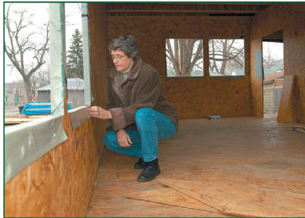
Demonstration House 1 construction showing a novel “studless” wall system of 1-1/2-in. OSB panels that will be covered by an exterior thermal and moisture management system.
