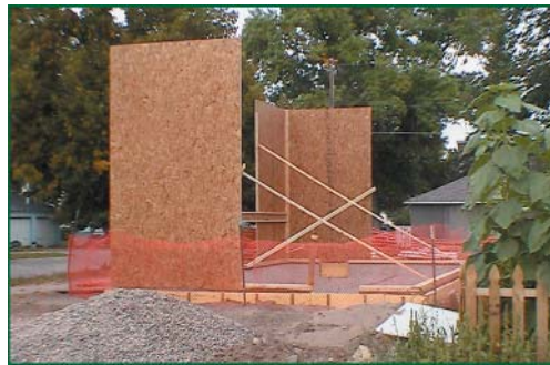
Erection of the SEP wall system on Demonstration House 2. The floor system will be installed next.
