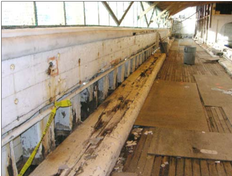
Starboard view of deteriorated waterway and main decking
