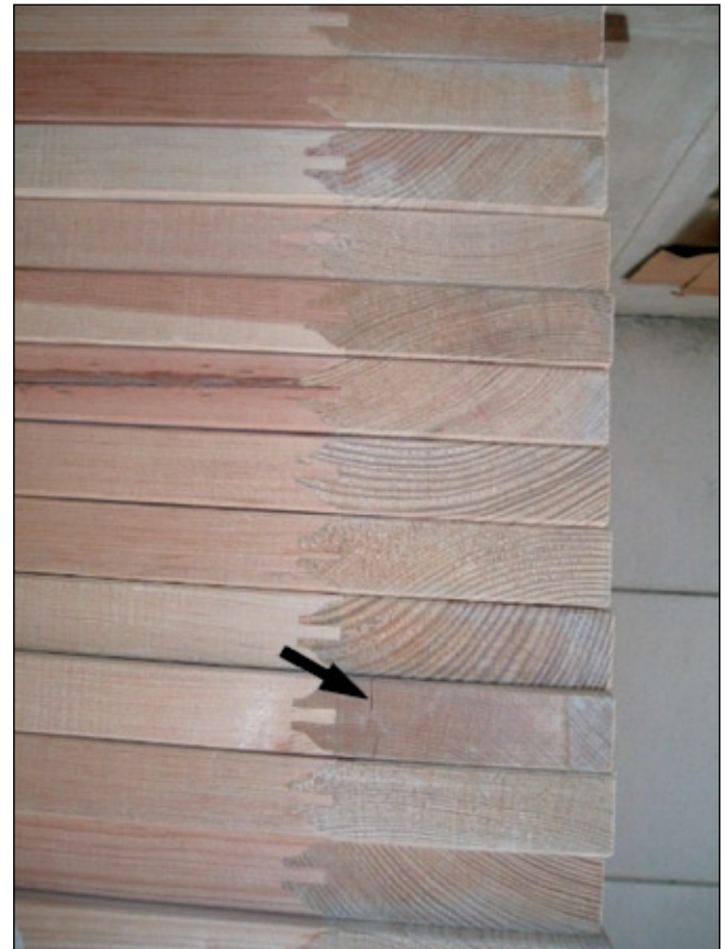
Figure 22—End checking on flat-sawn grain of unfinished door stiles.
