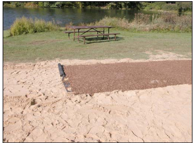
Figure 5—Termination of Soil-Sement portion of beach path. Geotextile fabric visible under completed SEWF surface.
