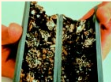
Zebra Mussel populations can completely restrict flows in intake pipes. Department of the Interior, United States Geological Survey, Photo by Don Schloesser
