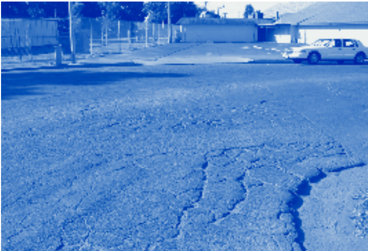
Typical street pavement failure area where numerous trench cuts have occurred over time.
