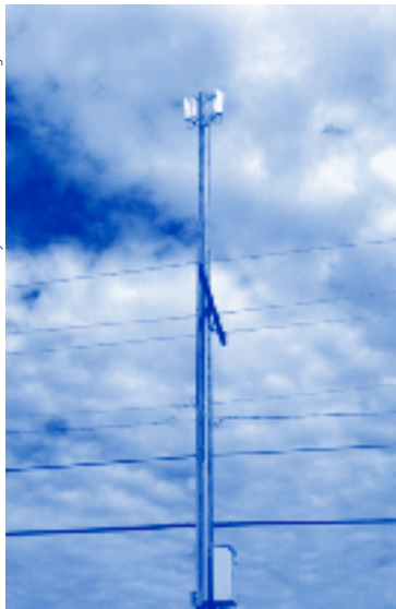
Broadband transmission equipment as seen on a telephone pole.
