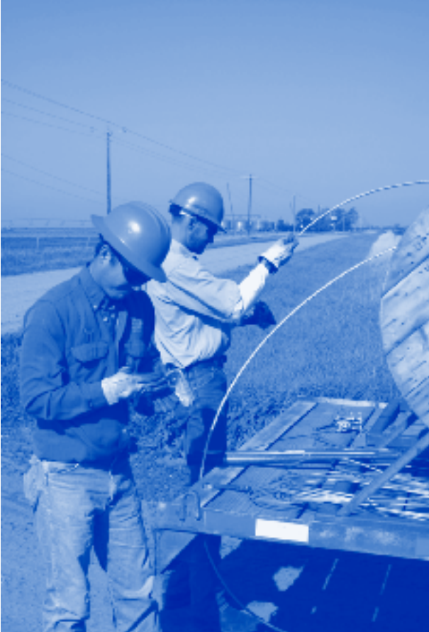
Lineman Steve Nelson, left, and Mark Thompson prepare to string wire for a new irrigation service in Holt County.
