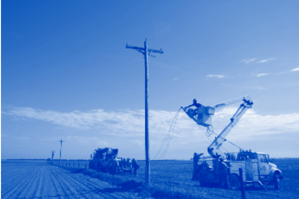
Shane Powell holds the arm on a bucket truck as he raises the wire conductor to be attached to the insulators.
