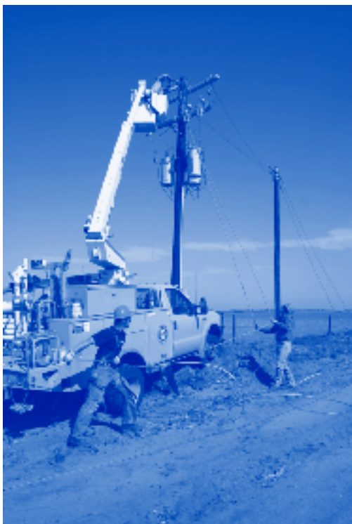
Lineman Jeremiah Krysl, in the bucket, connects the wire conductor to the crossarm as Steve Nelson, right, and Shane Powell, work to pull the slack from the line.
