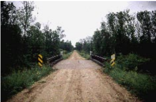
Figure 5—Ciphers bridge after 46 months in service: side view (top); end view (bottom).
