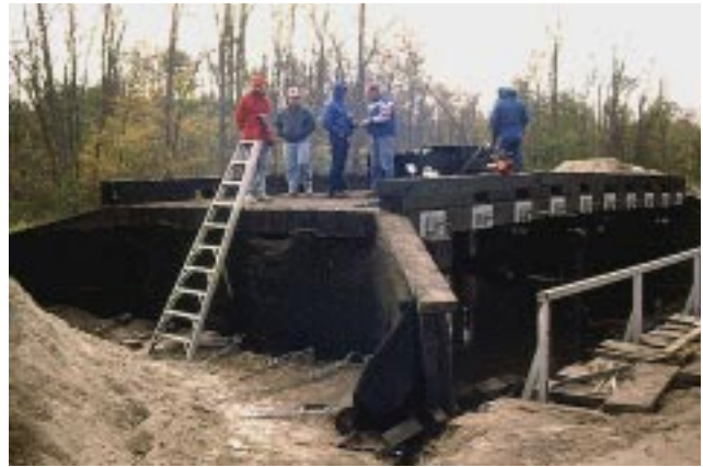
Figure 4—Ciphers bridge was prefabricated in two half-width panels that formed the deck after the initial bridge stressing.
