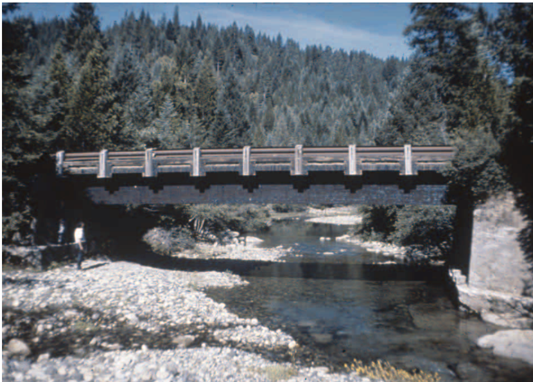
Figure 2—Oil-type preservatives are often used for treatment of glulam beams, such as in this bridge.
