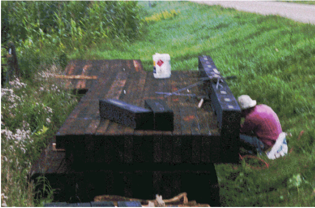
Figure 7— These bridge components are being bored and field treated off-site before being positioned over the water.
