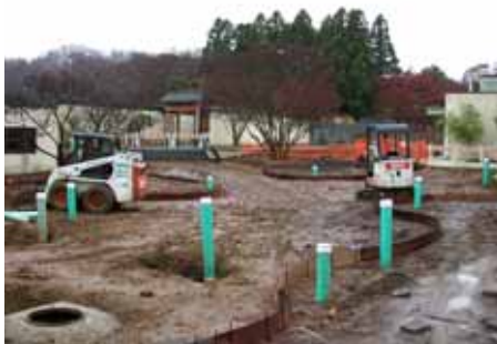
Construction of the new lower courtyard in the National Bonsai and Penjing Museum.
