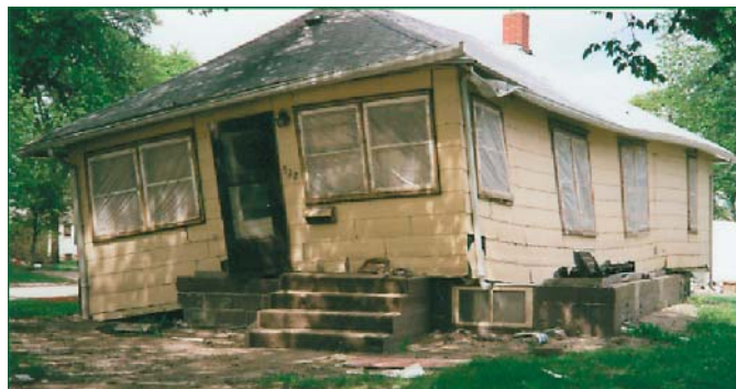
Post flood damage to a wood-frame house.
