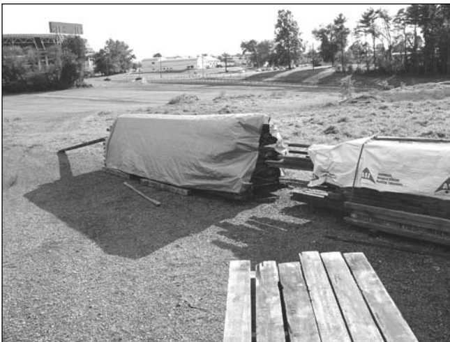
Figure 2—The lumber was covered with tarps open at the ends to allow air drying while preventing further wetting from rain.
