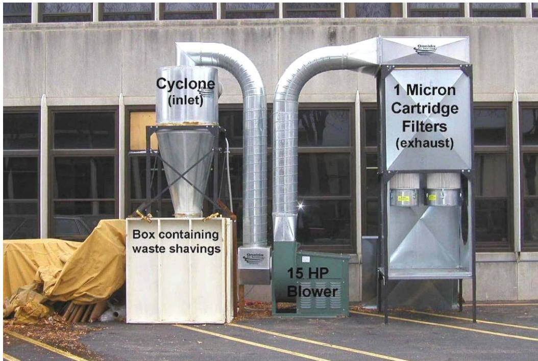
Figure 15. Oneida dust collection system as installed outdoors at FPL.
