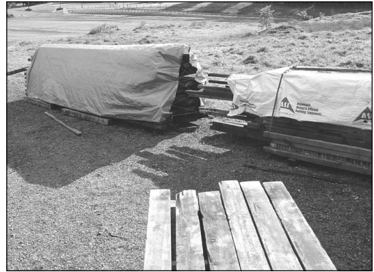
Covering the deconstructed lumber with tarps open at the ends allow for air drying while preventing further wetting from rain.
