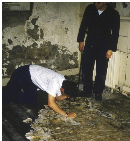
Inspectors check the underside of a wooden floor for fungal growth. The floor was located in a Scottish castle. The damp castle was an ideal location for fungal growth.
