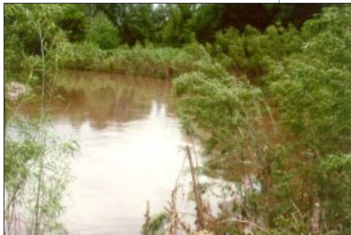
The Court Creek bank erosion site near Dahinda has averaged 2000 tons of sediment per year since 1940 (top). With funding from USCOE Waterways Experiment Station, biotechnical bank stabilization was completed in 1994 (center). The site has remained stable throughout a series of large floods (bottom).
