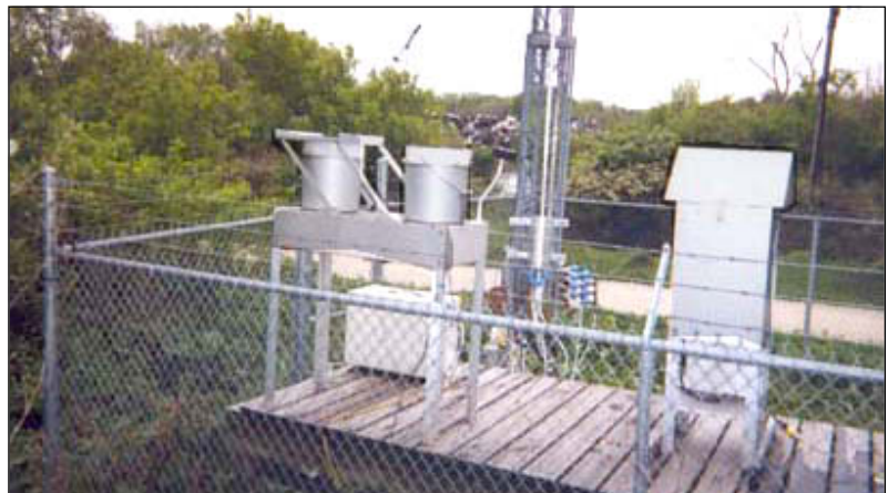
Air-quality sampling equipment at a site near Lemont detects salt particles in the air.
