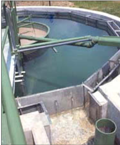
Small potable water treatment plants use an up-flow clarifier to remove dissolved solids.
