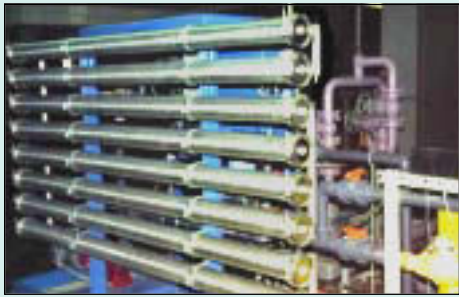
The IWTP also keeps existing state facilities up to date with current technology. This reverse osmosis equipment is used to pretreat boiler makeup at the Dixon Correctional Center.
