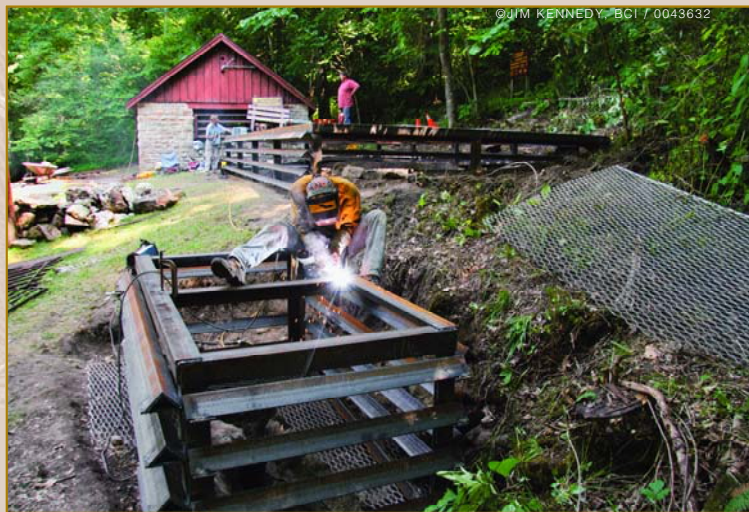
A welder works on a cupola gate Saltpetre Cave, one of four bat-friendly gates installed at this important Kentucky site.
