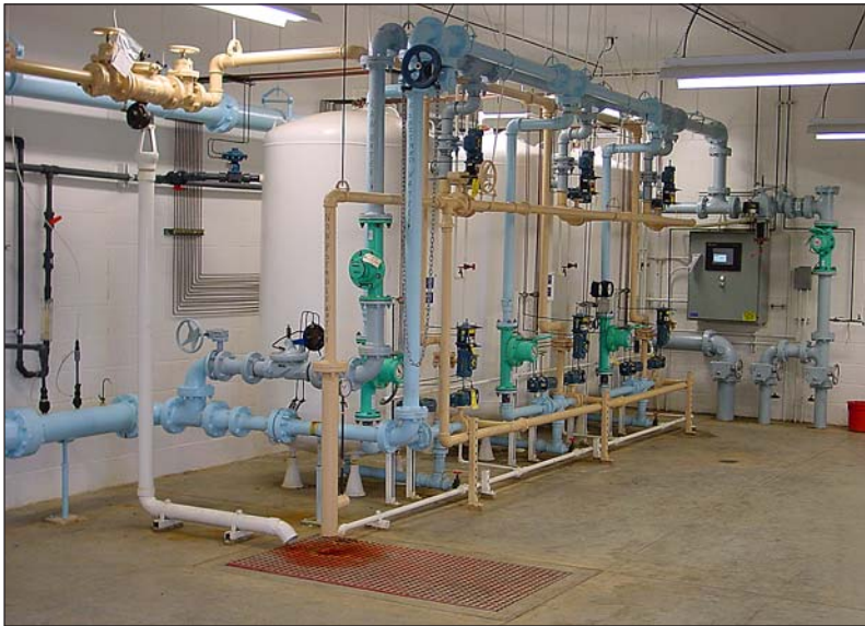
Dwight Correctional Center has three cold distribution water softeners.
