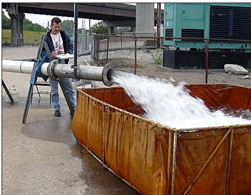
Mark Anliker records the pumping rate from an orifice tube during a step test of the IDOT dewatering well near East St. Louis.
