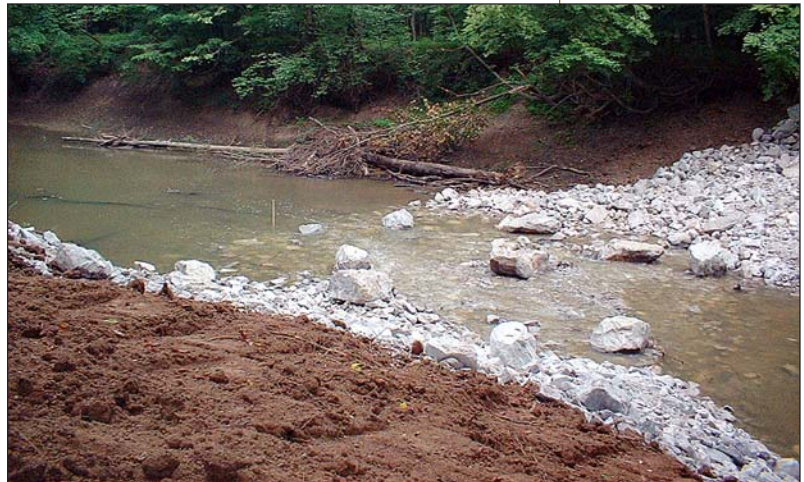
This is the Cache River site before (top), during (middle), and after (bottom) installation of riffle/pool restoration structures.
