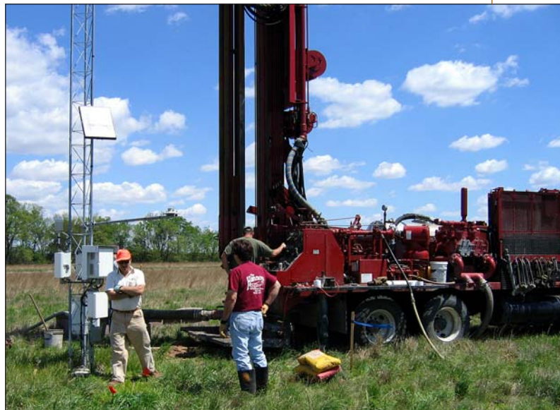
Under supervision of Bob Olson and Ken Hlinka (left to right) an Albrecht Drilling crew installs an observation well for the ICN site at Big Bend.
