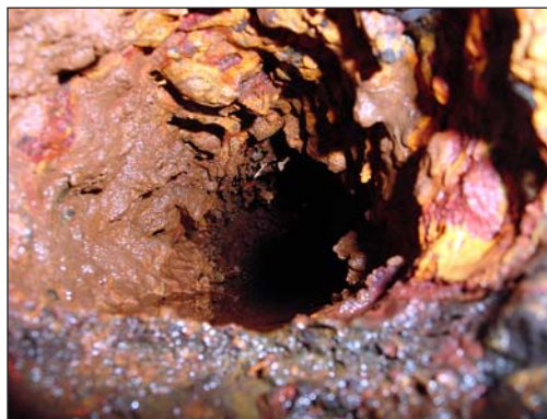
This close up shows scale deposits in a 4-inch diameter feedwater line at Western Illinois University.
